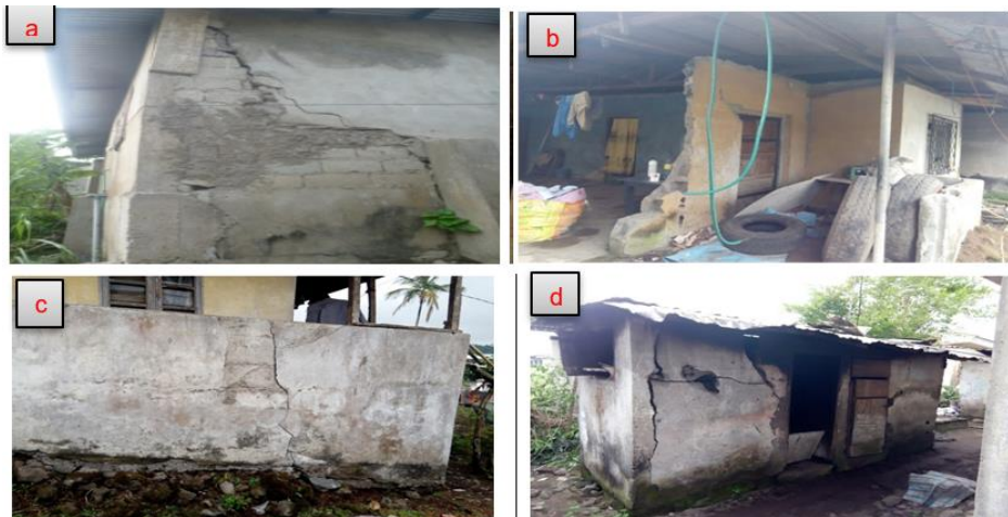
Fig. 8. Damaged buildings in Buea during the 1999 eruption at: a. Small Soppo, b. poto-poto quarter-Bokwango, c. Buea Town and d. Small Soppo
